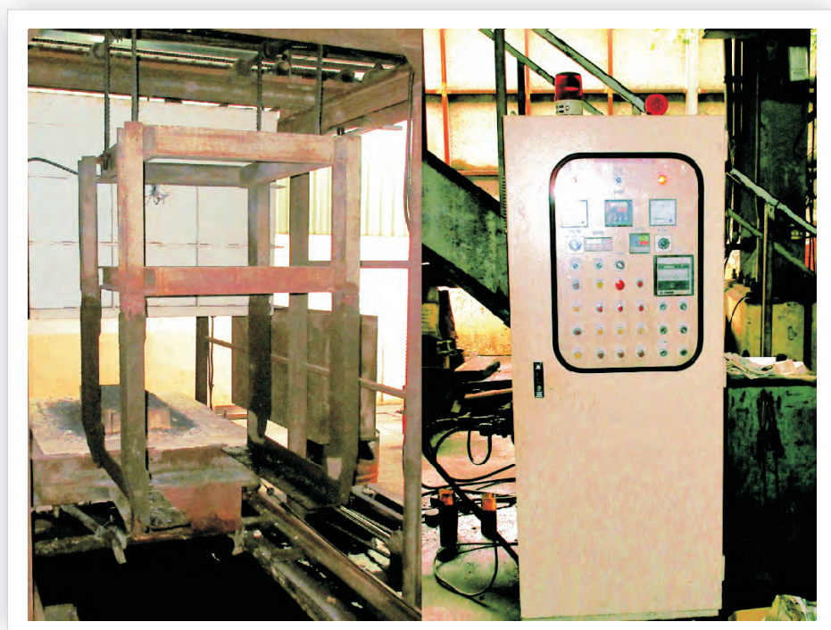
▼熱處理設備 FURNACE FOR HEAT TREATMENT
